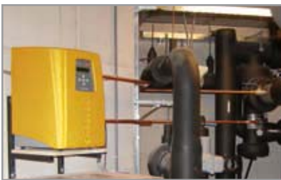
Occupants are happy now that the SpiroVent Superior S3 has been installed.
